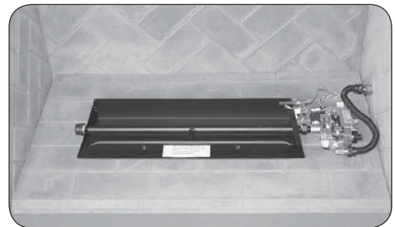
Fig. 18-2 Center burner in fireplace
